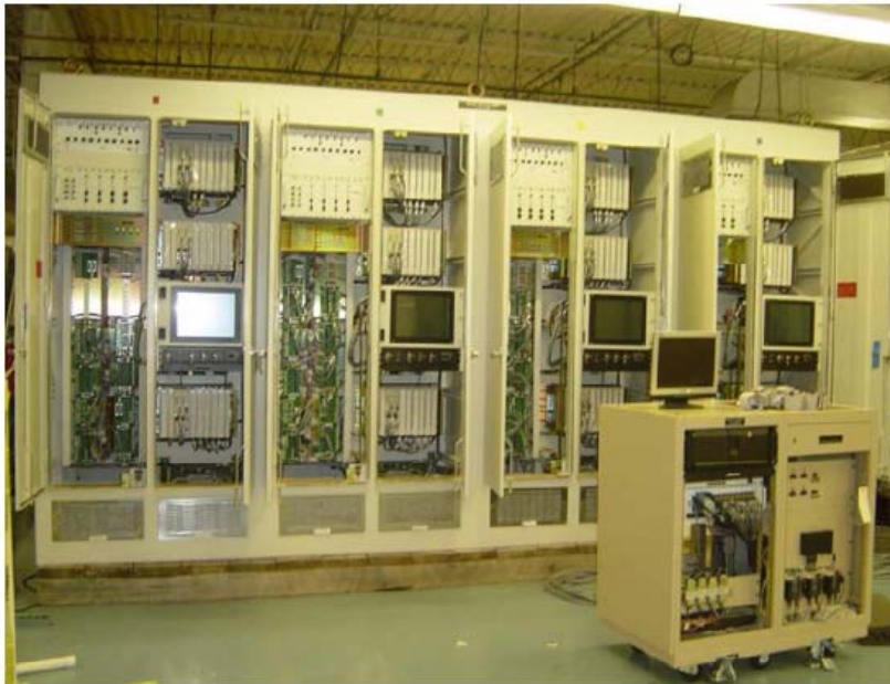
PLCs in cabinets (CPCS) - Westinghouse
