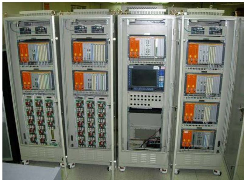
PLCs in cabinets (ESF-CCS)
